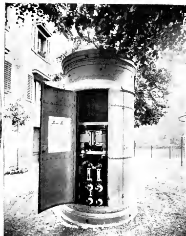
FIG. 7.—HIGH-TENSION SIDE OF TRANSFORMER HOUSE.
